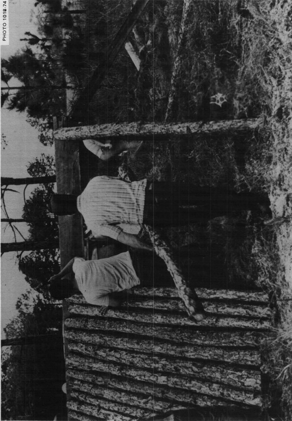
Fig. 5.46. Nailing a 9-ft roof pole to the ridge board. This photograph is misleading as regards the lower ends of the ridge poles; actually the ends rested against a 1 x 6 board placed against the outer side of the 6-in.-deep V trench that marked the edge of each shelter side wall.
